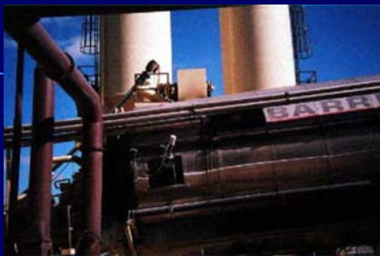
Double drum asphalt plant with 2 silos – one for hydrated lime & one for mineral filler
