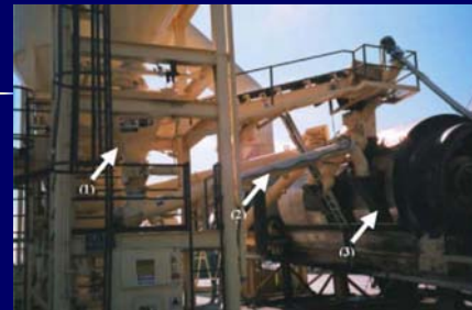
Weigh pot (1) dispenses lime through rotary vane feeder (2) and into outer shell (3) of double drum plant
