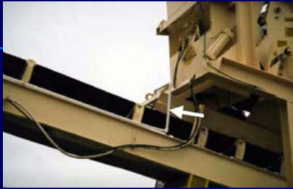
Water delivery system mounted over aggregate conveyor (see arrow)
