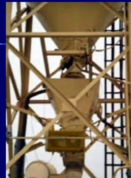
Hydrated lime is dispensed from the silo through a weigh pot
